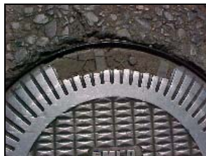
Cracked spill bucket lid
