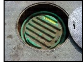
Circular steel sump lid pulled back to show the inner lid covering the turbine sump
