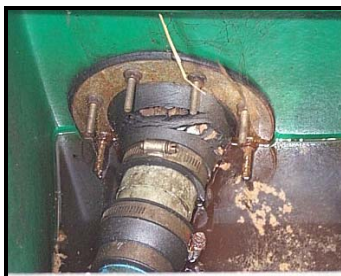
Sump penetration seals in poor condition
