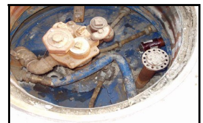
Flexible piping is kinked
