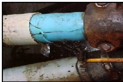
Flexible piping is cracked
