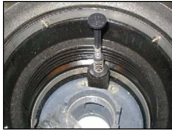
Spill bucket drain valve
