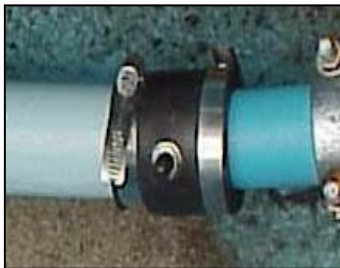
Test boot located in a sump
